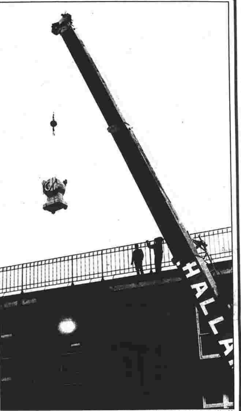
SAFE LIFT - A worker guides a 3,000-pound safe as a crane lowers it Monday from the Hartford Road offices of Fuss & O'Neill. The former Cheney Bros. safe will now make its home at the Lutz Children's Museum.
